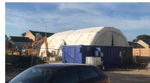
Figure 2 – Inflatable tent used to contain emissions.
