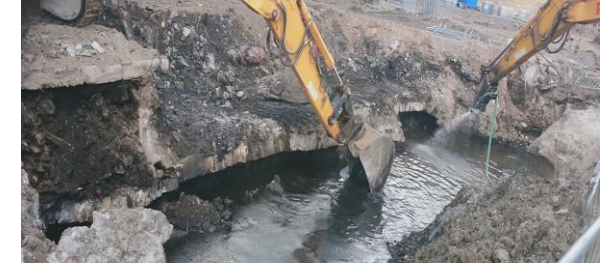
Removal of contaminated tunnel system prior to benching and reinstatement with remediated materials.
